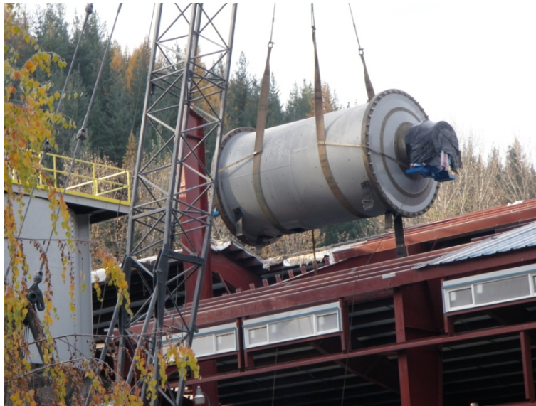
Figure 6. New grinding mill for New Jersey's mill at Kellogg, Nov. 2011.
